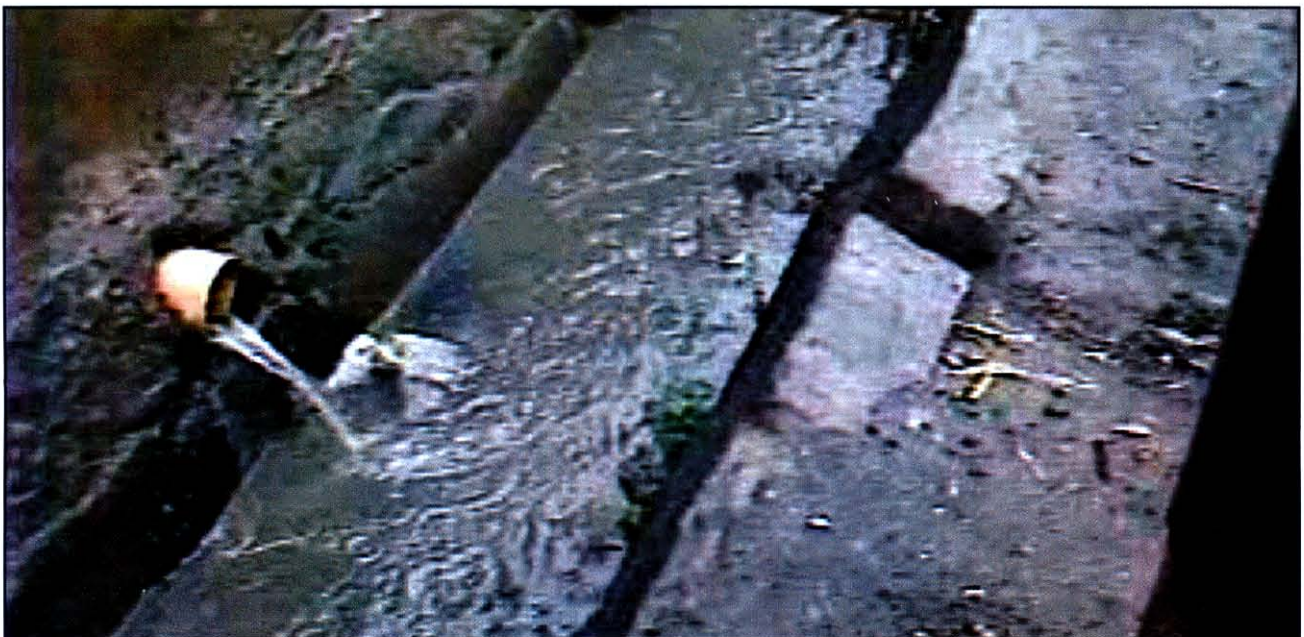
Picture 2: Photograph showing surface drainage channel with waste water draining into it and a 'clean' water pipe crossing through the channel.
