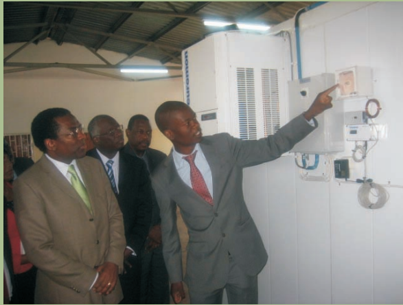
Mr Abrahams Mwanamwenge, NPO/LOG explaining to Dr Luis G. Sambo operations of the cold room facility in Ndola, Copperbelt Province
