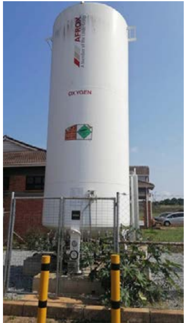
Figure 24: An oxygen plant at the Lubombo Referral Hospital
