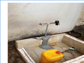
Figure 6. A typical example of one of the standpipes in Brookfields connected to the pipe network. The tap is closed after use by the people.
