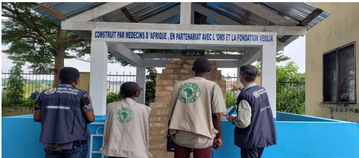
To ease the destruction of hazardous biomedical waste, WHO partnered with @FondationVeolia, @medecin-afrique to construct a biomedical waste incinerator at the M'filou hospital in Brazzaville/WHO-Marriane Tabi
